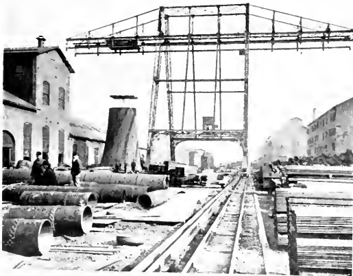
FIG. 7.—LARGE ELECTRIC GANTRY CRANE.
